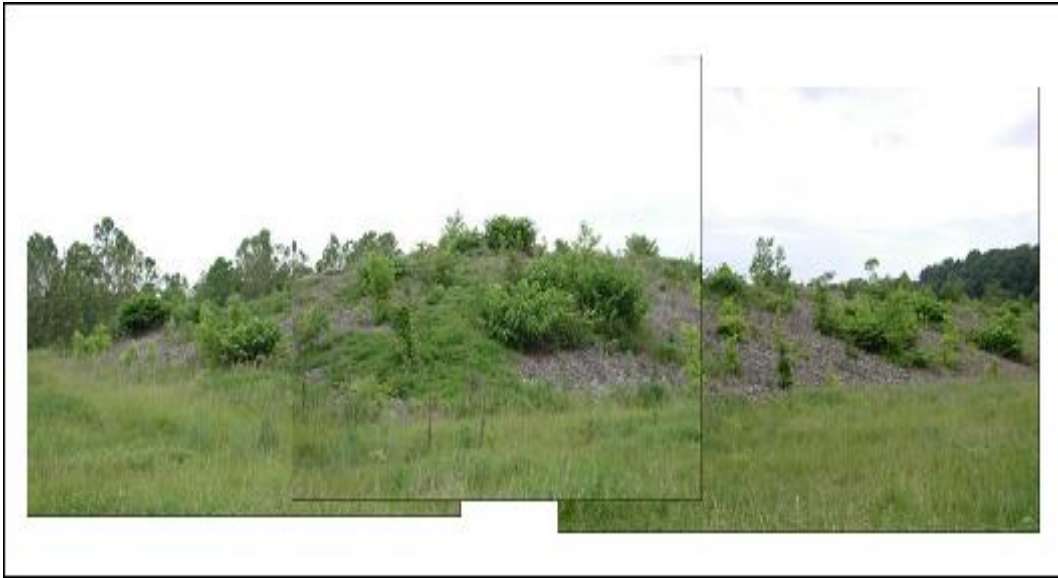
Figure 16. Photograph of Burrell, PA conventional cover demonstrating vegetation growth.
